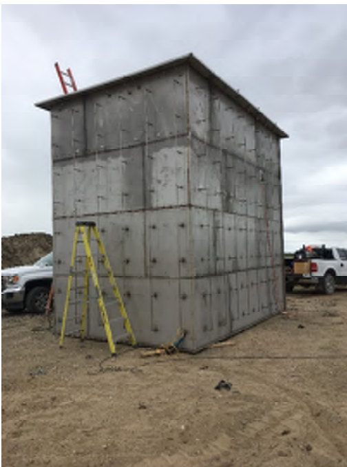
Ground Sump pit tank at Simplot
